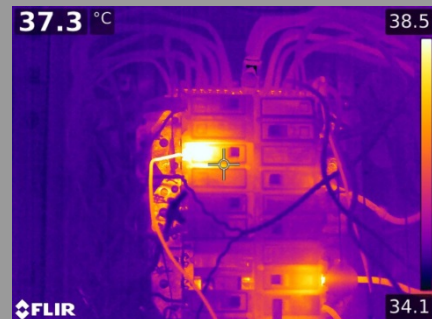
Failing connection in industrial breaker panel
